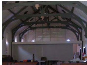
Hall - working out how the heating & lighting currently works in the hall (to be
